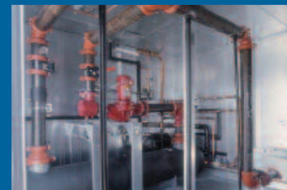
Typical Primary Pump and Inlet Strainer of a Primary/Secondary Pump Package
