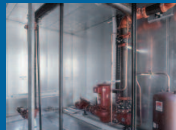
Typical Secondary Pump, Inlet Strainer and Expansion Tank of a Primary/Secondary Pump Package
